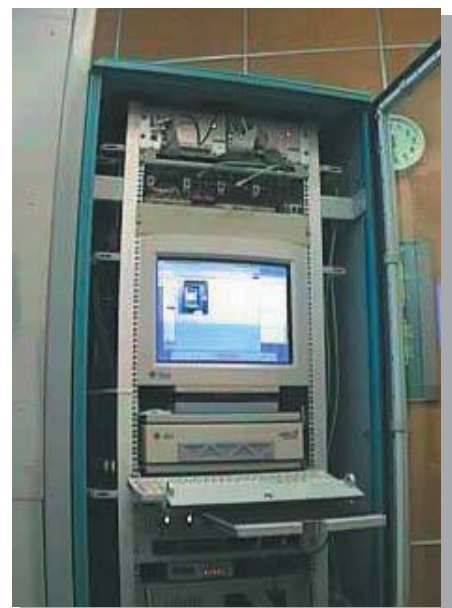
STCU Upgraded Information & Measuring System at the Chernobyl NPP
